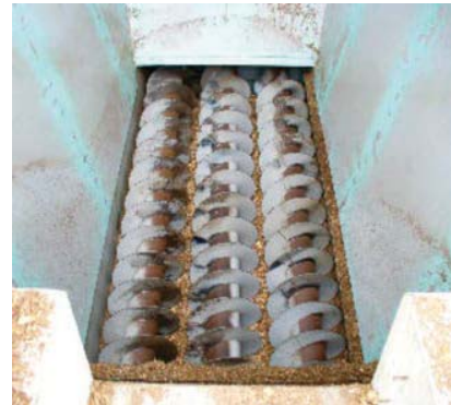
Mounting in discharge screw (wood-fired power plant)
